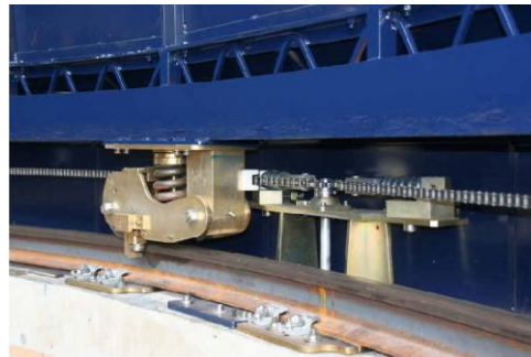
Figure 7. Guiding module of the dome. The rotation is obtained with a 30 meters chain and an asynchronous motor located downstairs
